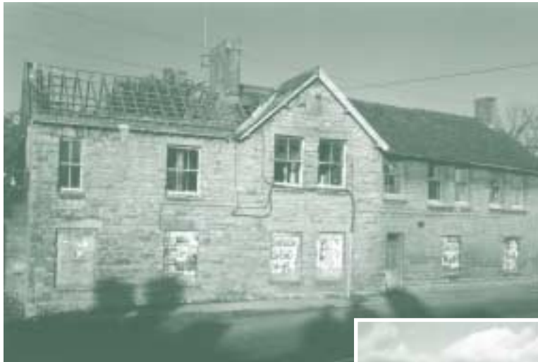
Above and right: The Morlands site between Glastonbury and Street.
